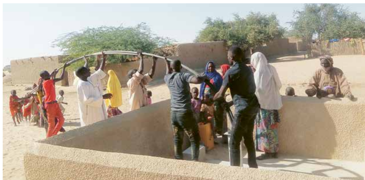
A new hand pump has been installed in Laouré Blabrim village in Niger and the first villagers are able to access clean drinking water.
